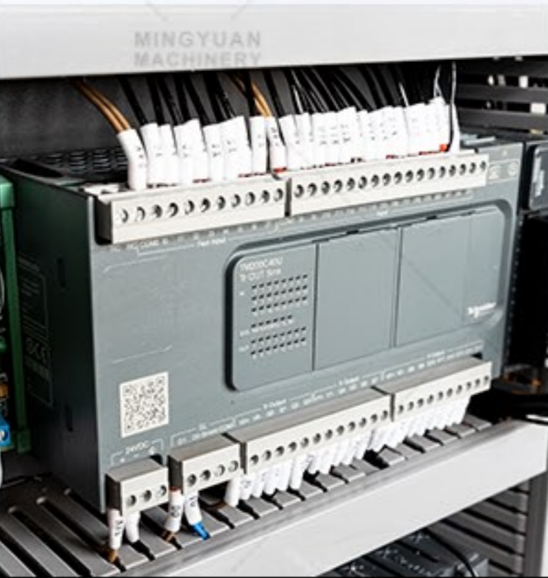
Schneider PLC Controller
